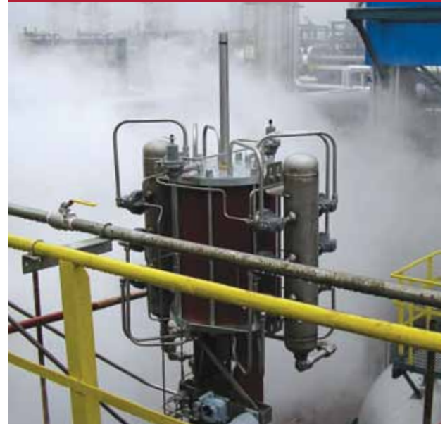
SVI II AP on steam conditioning valve
